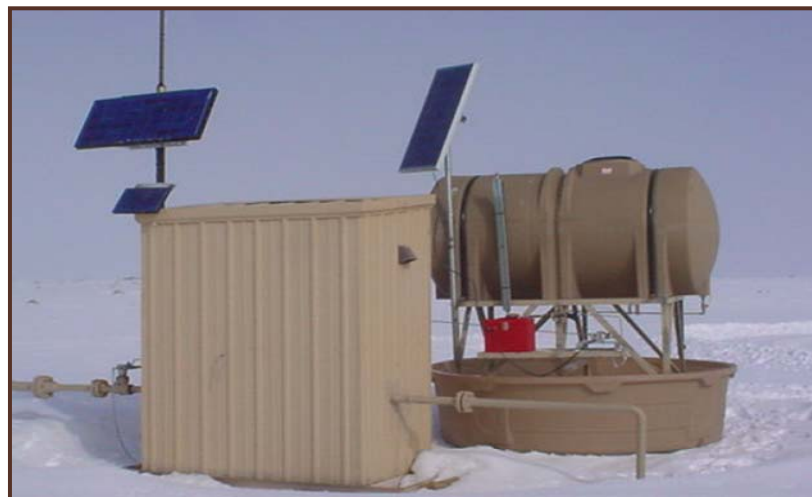
Source: Anadarko, Solar chemical pump - 5 - pumps
