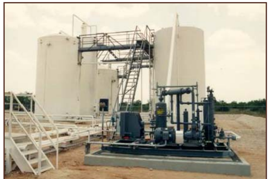
- 4 - Source: Hy-Bon Engineering, VRU
