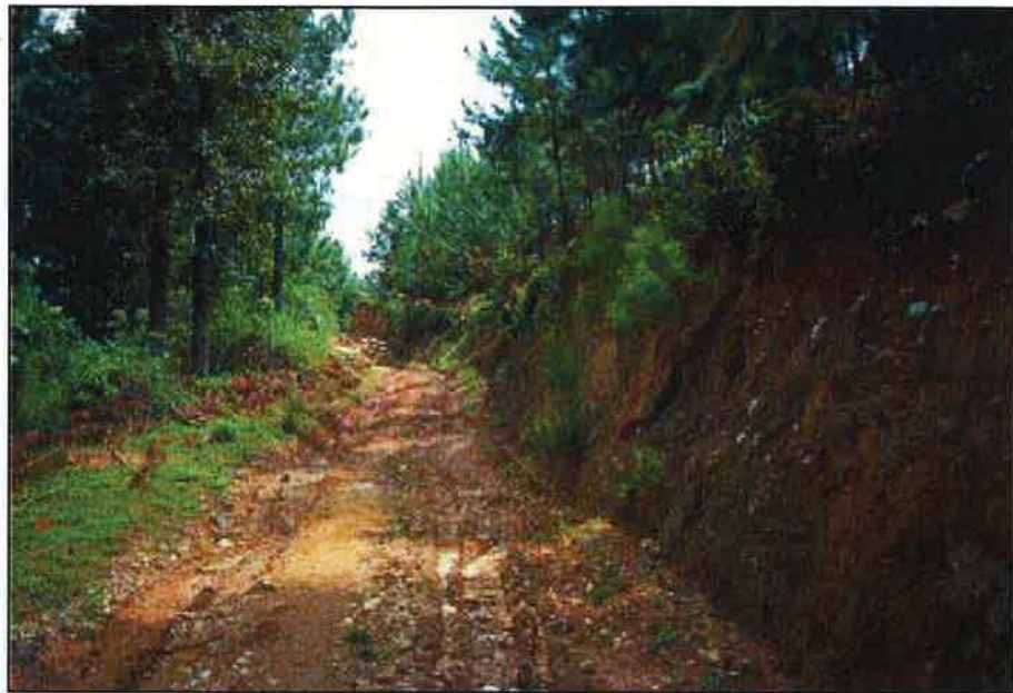
Photo 12.1 A rutting road caused either by soft subgrade soil or inadequate road drainage (or both).
