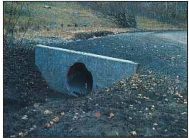
Photo 4.6 A well designed and installed culvert with head walls for efficiency and fill protection.
