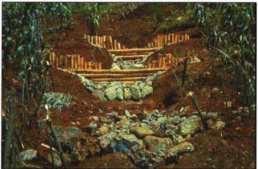
Photo 14.4 Construct debris retention and gully control structures with a notched wier to keep flow over the middle of the structure, add scour protection at the outlet of each structure, and key the structures into the firm soil banks.
