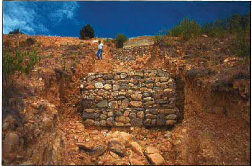
Photo 14.3 An expensive but failed gabion gully control structure that was not properly keyed into the banks of the gully. Further, the flow was not kept over the protected middle of the structure.
