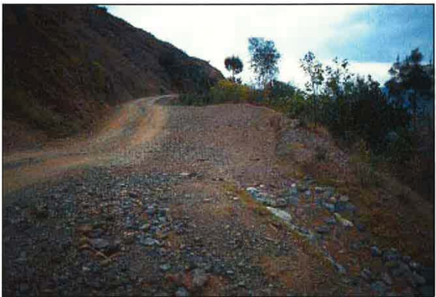
Photo 7.2 Use rolling dip (broad-based dip) cross-drains to move water off the road surface efficiently and economically, without the use of culvert pipes. Rolling dip cross-drains are not susceptible to plugging.
