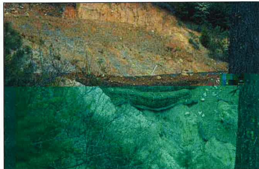
Photo 11.12 A gabion retaining structure which will fail soon due to lack of a suitable foundation. All retaining structures, either mechanically stabilized earth (MSE) walls or gravity walls, require a good foundation .
