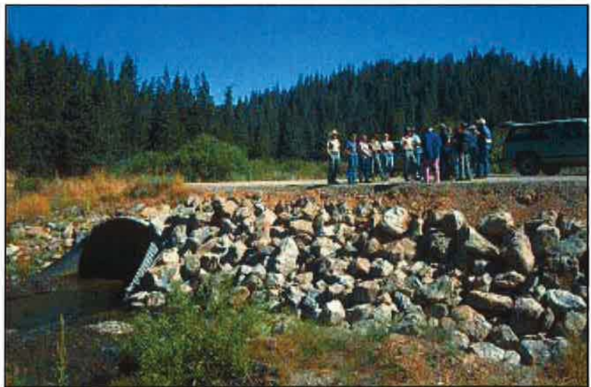
Photo 8.4 A structural plate arch pipe culvert with stream bank protection using large rock riprap placed upon a geotextile filter layer.
