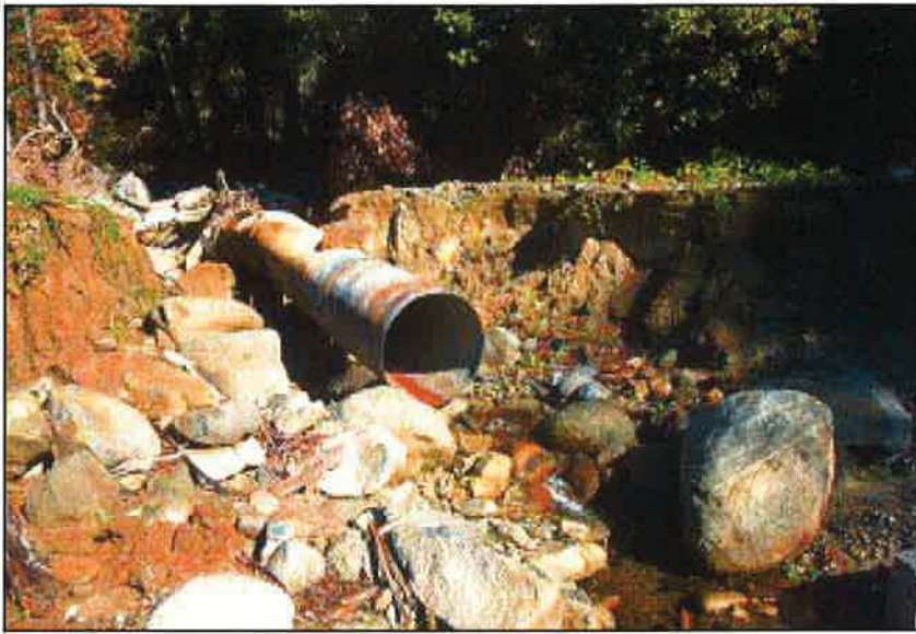
Photo 8.2 A culvert failure caused by insufficient flow capacity or inadequate pipe size to pass the debris (boulders) moving through the drainage.
