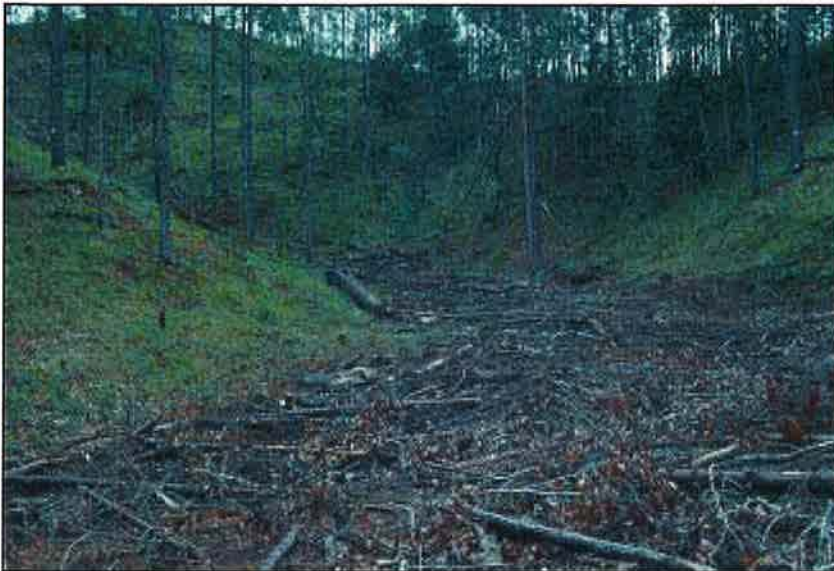
Photo 13.4 A disturbed work area covered with woody material such as brush from clearing or logging slash for erosion control . Ensure that the material is well mashed onto the ground.
