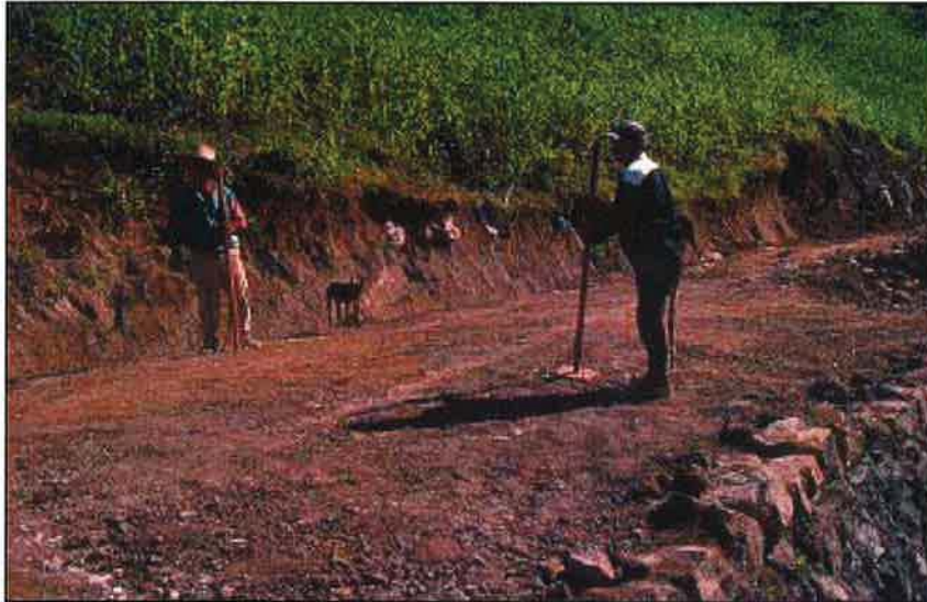
Photo 11.6 Simple hand compaction behind a low rock wall. Compaction is important behind any retaining structure or fill. It can be achieved by hand or, preferably, using equipment such as a wacker or small compactor.
