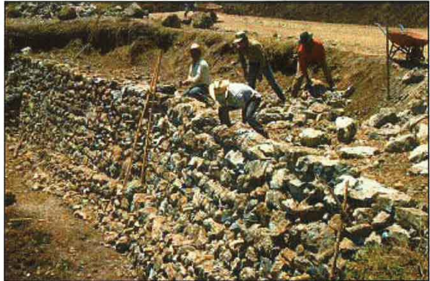
Photo 11.8 Use physical slope stabilization methods, such as retaining walls, reinforced fills, or rock buttresses where necessary in areas of space limitation on steep slopes.
