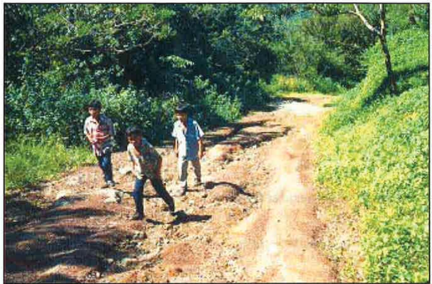
Photo 2.4 Adverse environmental impact from road surface erosion caused by steep road grades and insufficient cross-drains. This road is also difficult to maintain.
