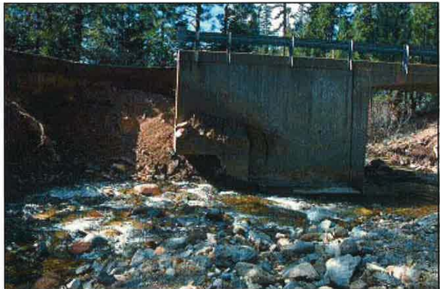
Photo 10.3 Scour is one of the most common causes of bridge failure. Use an opening wide enough to minimize constriction of the natural channel. Locate the bridge foundation on bedrock when possible, or below the depth of scour, and use stream bank protection measures such as riprap.
