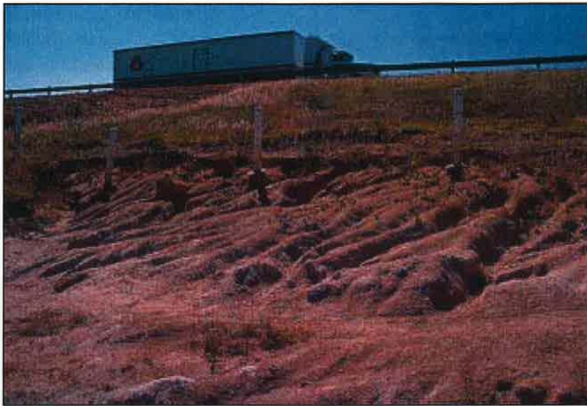
Photo 13.2 Erosion on a slope adjacent to a highway due to lack of vegetation or poor land use practices. Note that vegetation is preventing erosion next to the highway.
