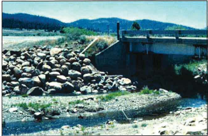
Photo 10.4 Concrete structures have a long design life and are typically very cost-effective for long bridge spans. Medium-length structures often combine a concrete deck placed upon steel girders. Use bank protection, such as riprap, to protect the entrance and outlet of structures.
