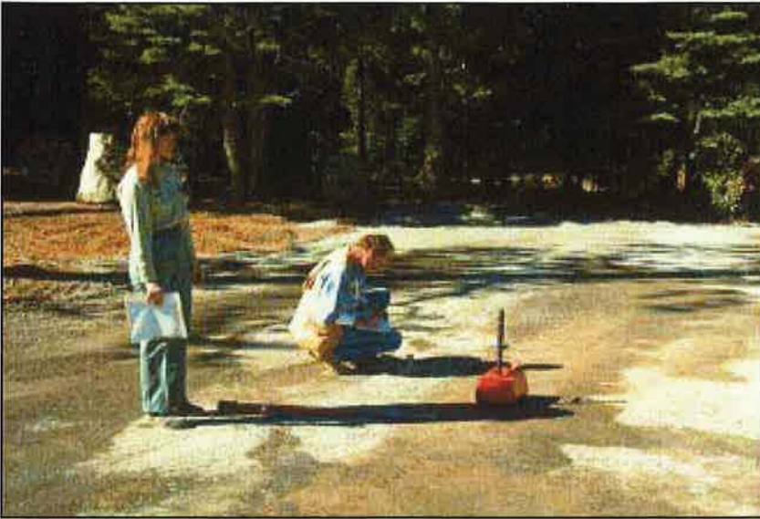
Photo 12.6 Here, a “nuclear gauge” is being used to check the density of aggregate. Use project construction quality control, gradation and density testing, etc., as needed to achieve the desirable materials properties for the project.
