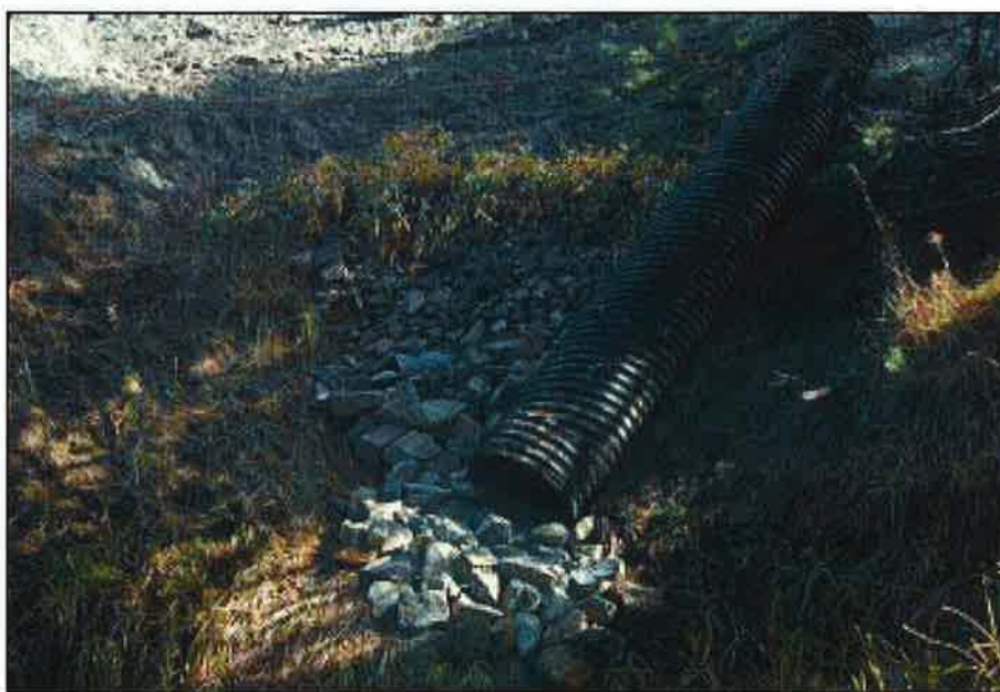
For small watersheds (up to 120 hectares) pipe size can be estimated using Table 8.1 (if better local data is not available). For larger drainages, specific site hydrologic and hydraulic analyses should be done. These analyses must consider the watershed and channel characteristics, high water levels, local rainfall data, and other available flow information (see Chapter 5, Chapter 6, and Chapter 7- Natural Stream Crossings). Photo 8.1 Protect the outlet of culverts against erosion. Graded riprap is commonly used for this purpose.
