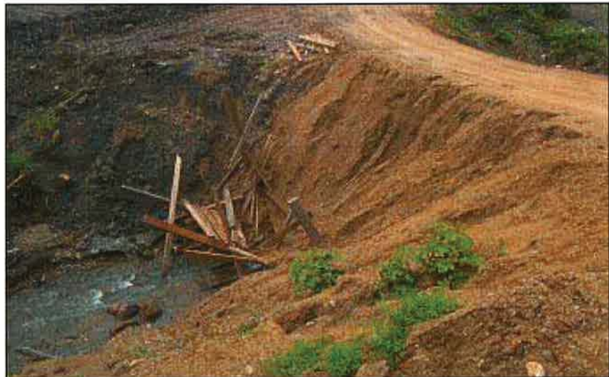
Photo 11.4 Avoid loose, over-steep fill slopes (steeper than 1 1/5:1), particularly along streams and at drainage crossings.
