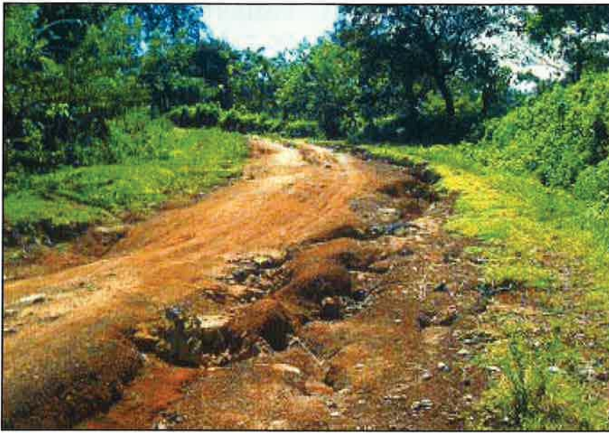
Photo 1.2 A poorly drained road that has a rough driving surface for the users, it is a source of sediment, and it is relatively expensive to maintain.
