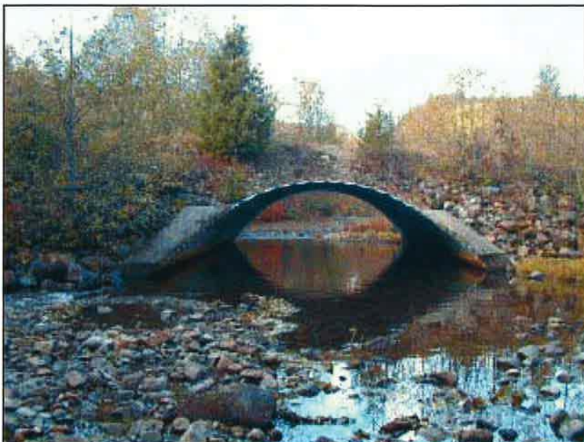
Photo 2.3 A bottomless arch pipe culvert that spans the active stream channel and doesn't constrict the flow, maintains a natural stream bottom, and helps promote fish passage. (Photo provided by S. Wilson-Musser)
