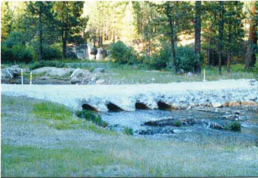
Photo 9.2 A vented ford, using multiple culvert pipes to handle low flows through the pipes, yet allow major flows and debris to overtop the entire structure.
