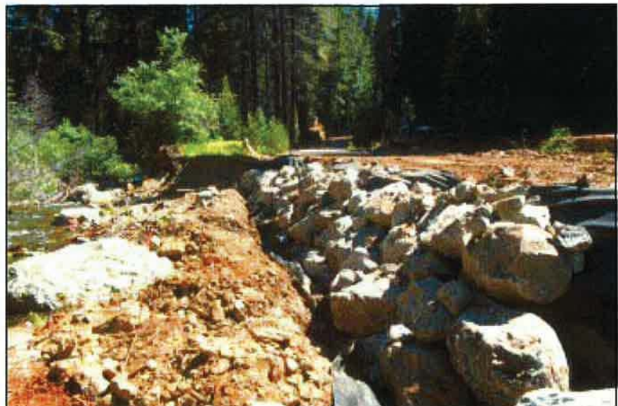
Photo 6.7 Riprap with a geotextile filter backing are being used to protect the road from high water flows. Note that the road is poorly located so close to the stream!
