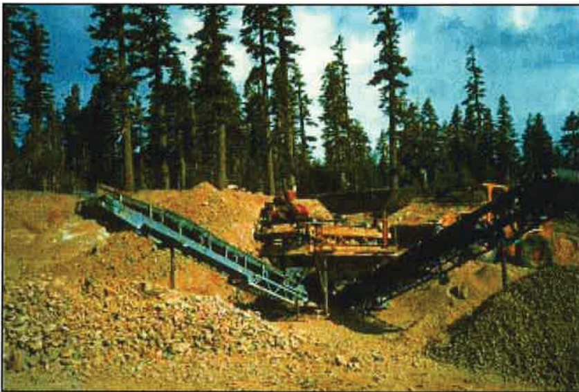
Photo 12.10 Quarries and borrow sites (materials sources) can provide an excellent, relatively inexpensive source of project materials. A site may require simple excavation, screening, or crushing to produce the desired materials. Control use of the area with a Pit Development Plan.
