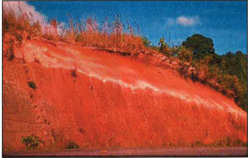
Photo 11.2 Construct cut slopes at a 3/4:1 or flatter slope in most soils for long-term stability. In well-cemented soils and rock, a 1/4:1 cut slope will usually be stable.
