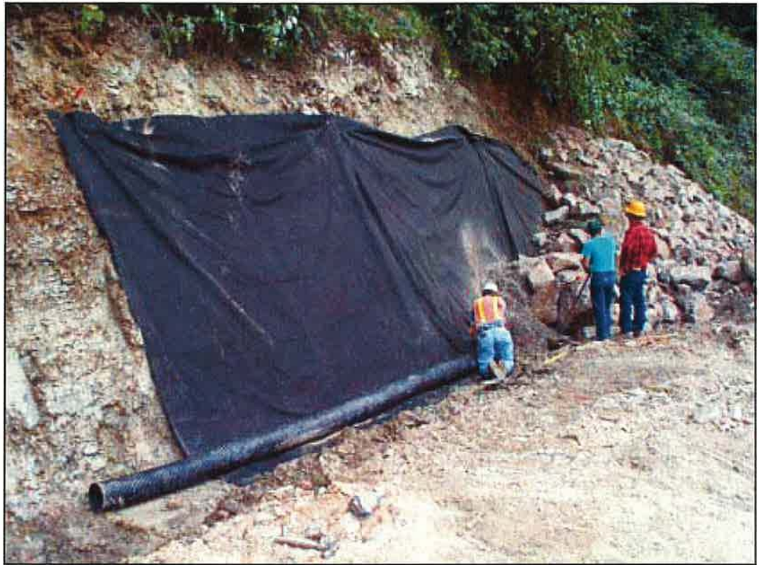
Photo 6.5 A filter cloth (geotextile) backing behind a loose rock slope buttress to provide a filter for drainage and to prevent movement of fine soil into the rock. (Photo by Richard Van Dyke)
