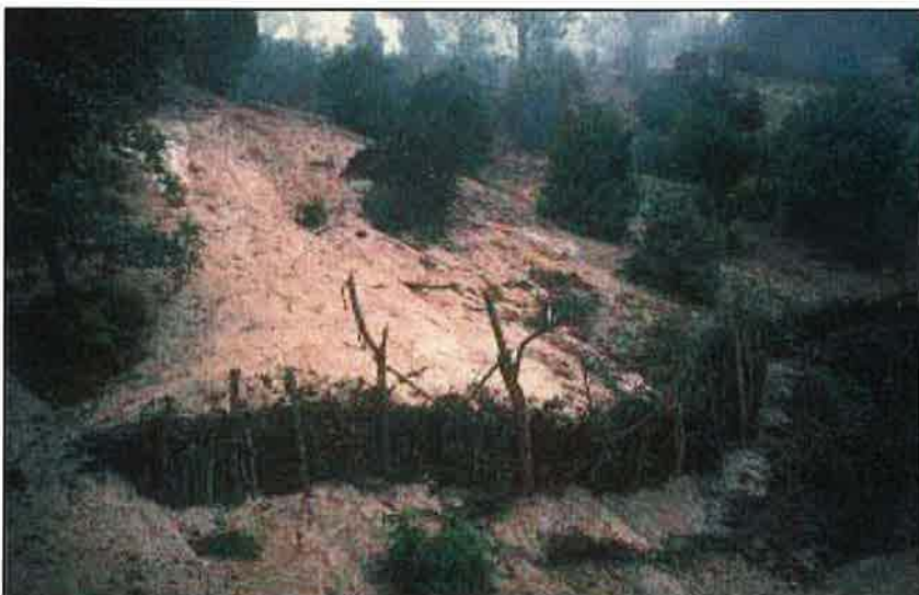
Photo 13.6 Sediment control fences (silt fences), live vegetative barriers, or brush fences can all be used to control sediment movement on slopes (also see Photo 6.6 ).
