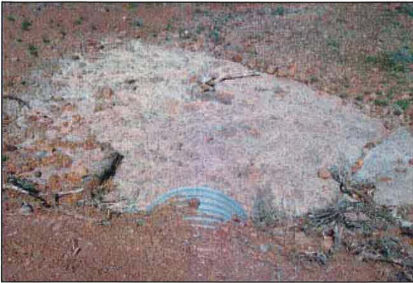
Photo 7.5 Protect the outlet of culvert pipe and rolling dip cross-drains with riprap or a masonry splash apron, or choose areas of bedrock or dense vegetation.
