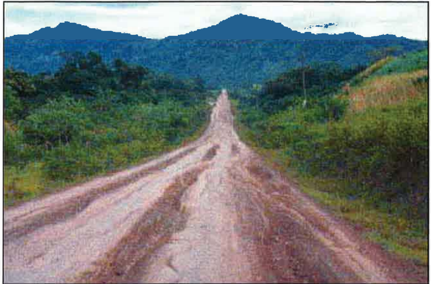
Photo 12.3 A road in need of maintenance and surfacing. Add roadway surface stabilization or do maintenance with grading and shaping of the surface to remove ruts and potholes before significant road damage occurs, to achieve good road surface drainage, and to define the roadbed.
