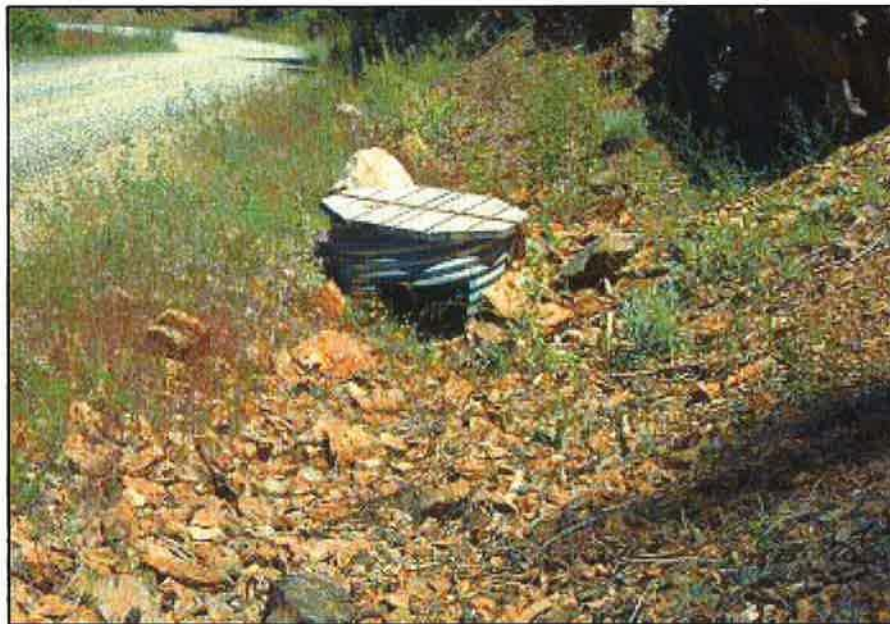
Photo 7.7 A rock armored ditch and metal drop inlet to control the water and prevent down-cutting of the ditch.
