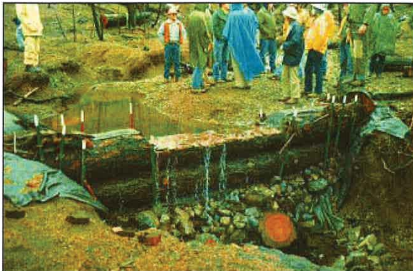
Photo 14.2 Logs being used to build gully stabilization structures in a fire damaged area. Physical or vegetative dams (dikes or debris retention structures) may be used to control sediment and stabilize gullies. Prevent water concentration before gullies form.
