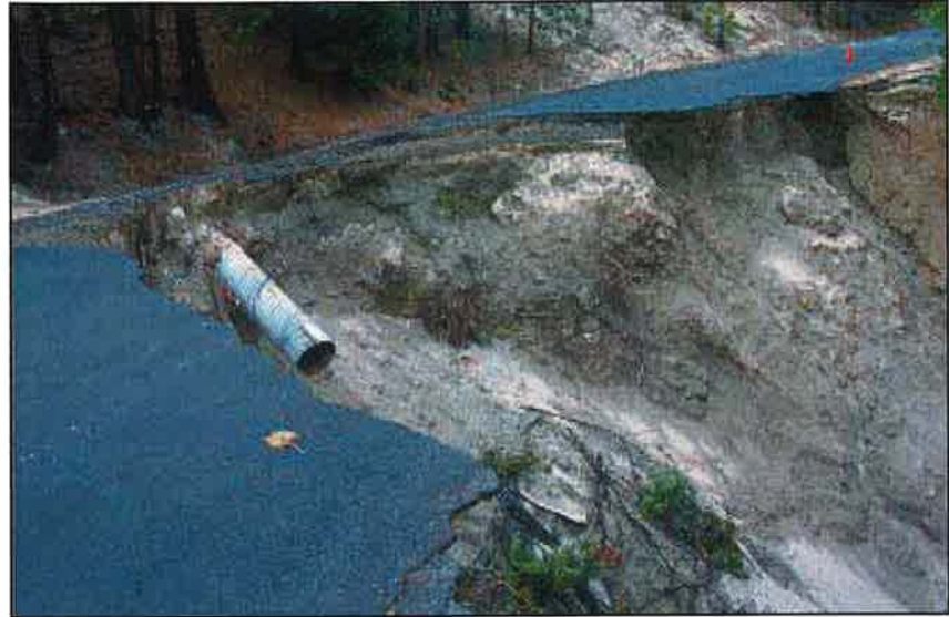
Photo 11.10 A road fill failure in steep terrain which now needs either a retaining structure or a large road cut around the failure.
