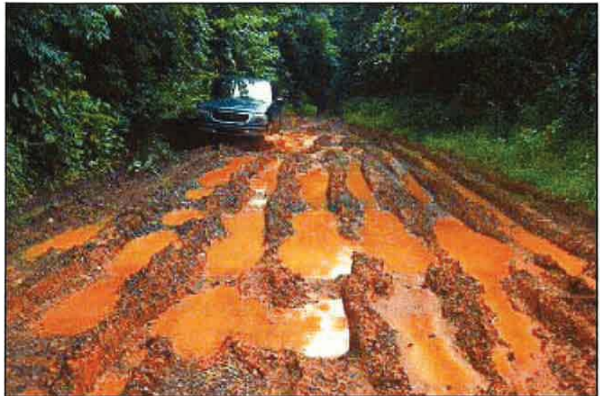
Photo 4.8 Avoid construction and other road activities during wet periods when possible. Alternatively, add drainage and surface stabilization to the roadway in weak soil areas for all-weather use.
