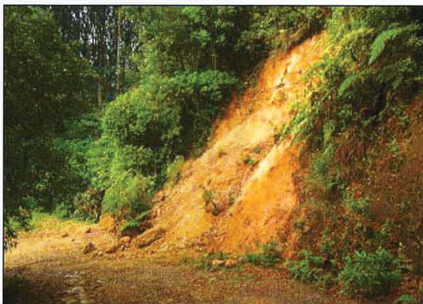
Photo 11.1 Over-steep slopes, wet areas, or existing slide areas can cause instability problems for a road and increase repair and maintenance costs, as well as sediment production.
