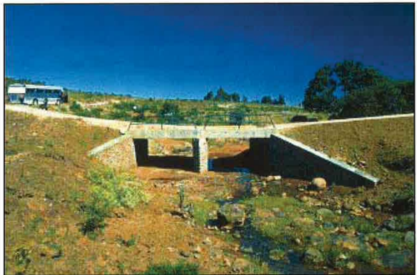
Photo 8.3 Install masonry/concrete box or metal culverts with a large enough size (capacity) to safely pass the anticipated design flow (typically a 20- to 50-year recurrence event), based upon hydrological analysis. Use headwalls and wingwalls whenever possible.
