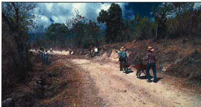
Photo 4.7 Use the road construction techniques that are most appropriate and cost-effective for the job and geographic area. Hand labor versus equipment depends on labor costs, equipment availability, and production rates.
