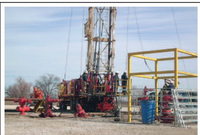
In this photo of a Devon Energy Barnett Shale multiwell pad site in the Barnett Shale play near Haslet, Tx., a wellhead is being put into place next to two existing wellheads, while another waits to be installed.
