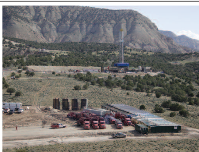
Williams Production RMT Company is using centralized pads to hydraulically fracture multiple tight gas sands wells on 10-acre spacing from a single central pad location in the Piceance Basin in Colorado. Working on as many as 22 wells simultaneously, the company has fractured as many as 140 wells from a centralized location, some as far as three miles away.
